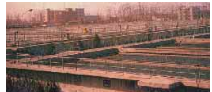
The Gao Bei Dian conventional primary plus activated sludge treatment plant serving a quarter of Beijing, China.
