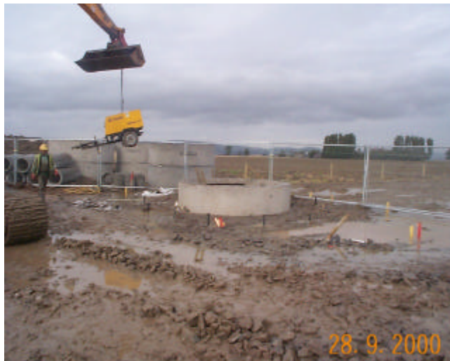
Figure 2.8. The lagoon pumping station
