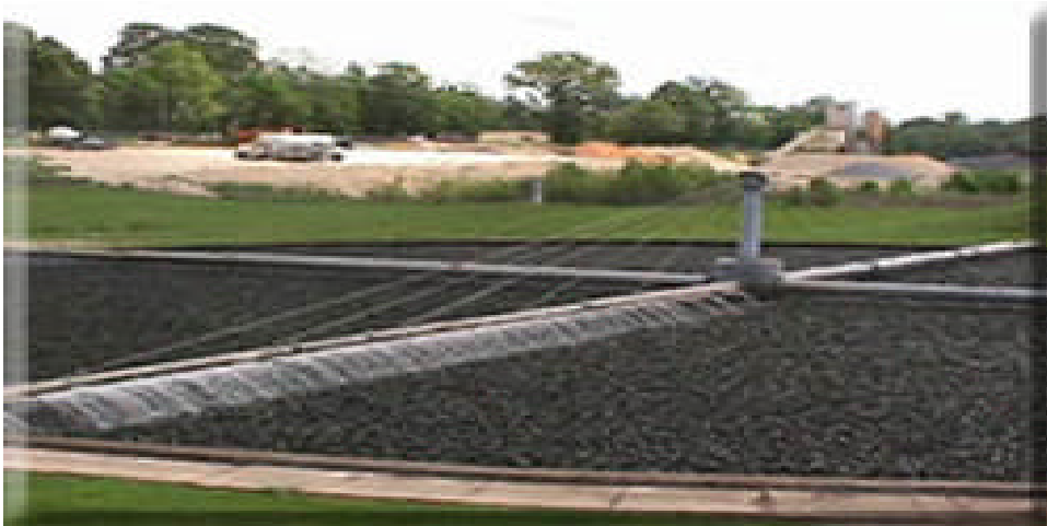
Figure 2.3. Trickling filter showing the distribution arm and media (from: http://www.vicksburg.org/pages/wastewater/photos.htm )
