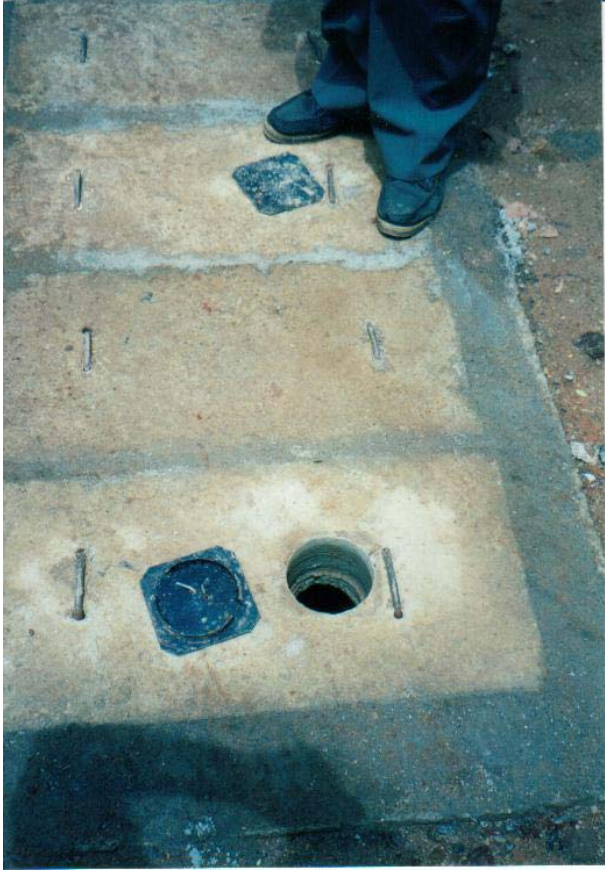
Plate 5-1. A typical inspection port.
