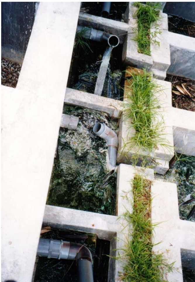
Plate 4-10. The effluent discharge elbows in a poor state of repair.
