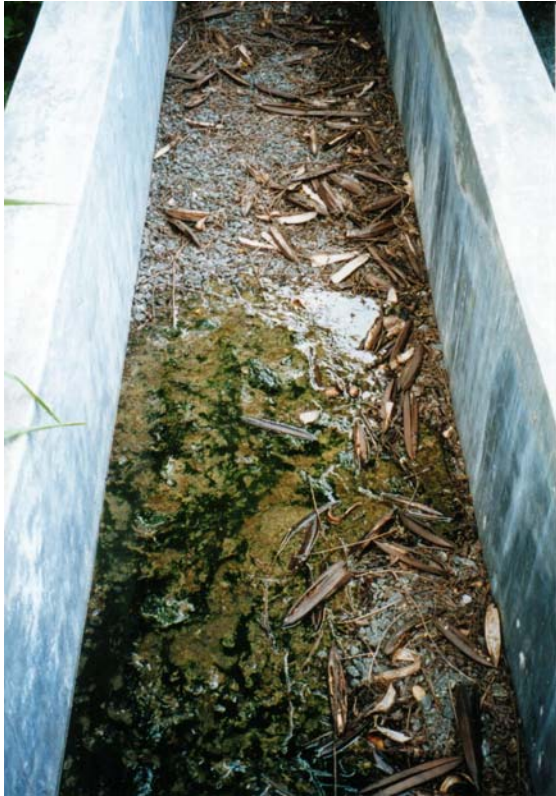
Plate 4-5. An unvegetated reed bed channel with inlet zone clogging.
