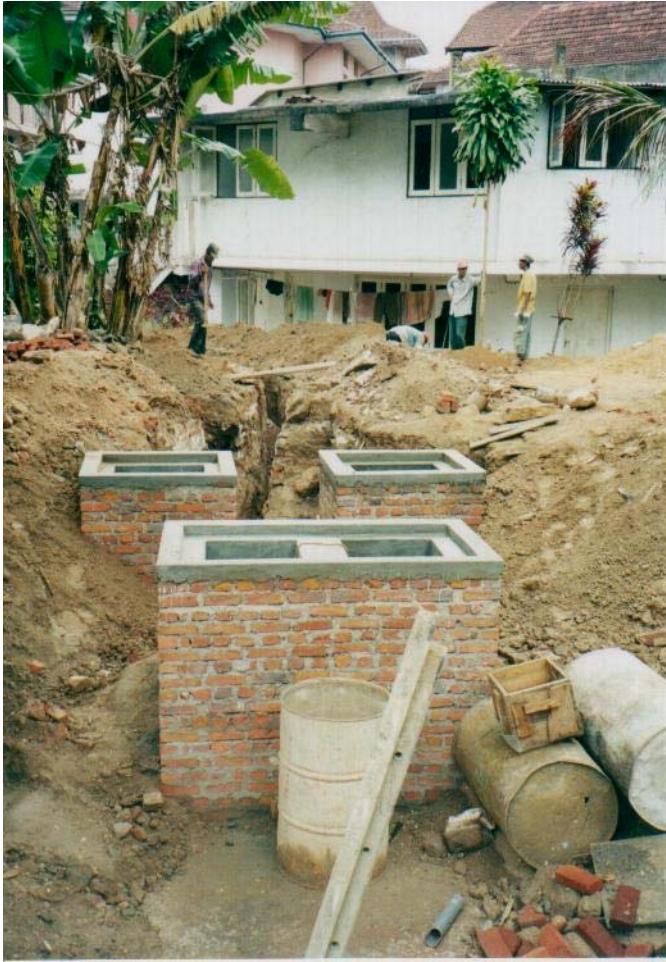
Plate 3-52. The raised access manholes of the septic tank-anaerobic filter.
