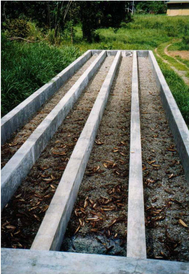
Plate 3-48. One of the reed bed stages at Akbar-Nell, soon after construction.
