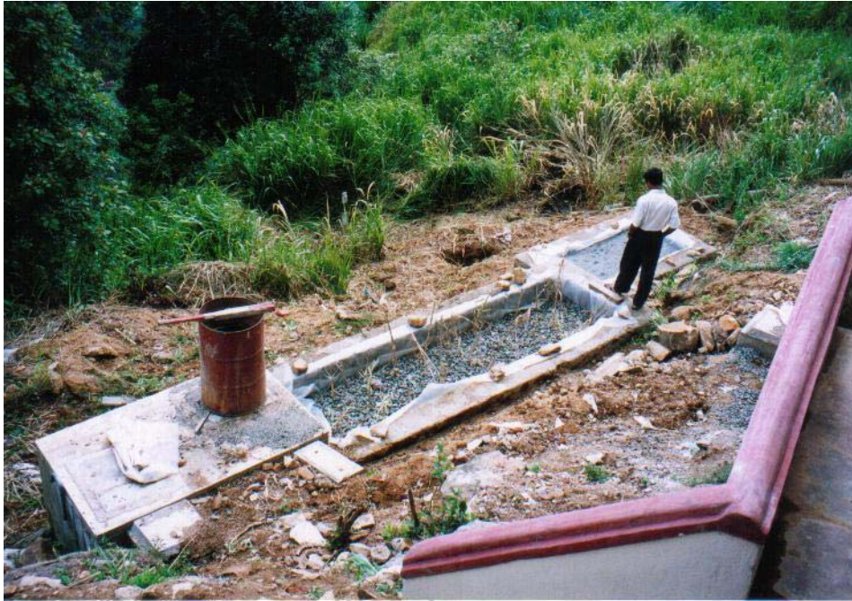
Plate 3-37. The constructed treatment system prior to commissioning
