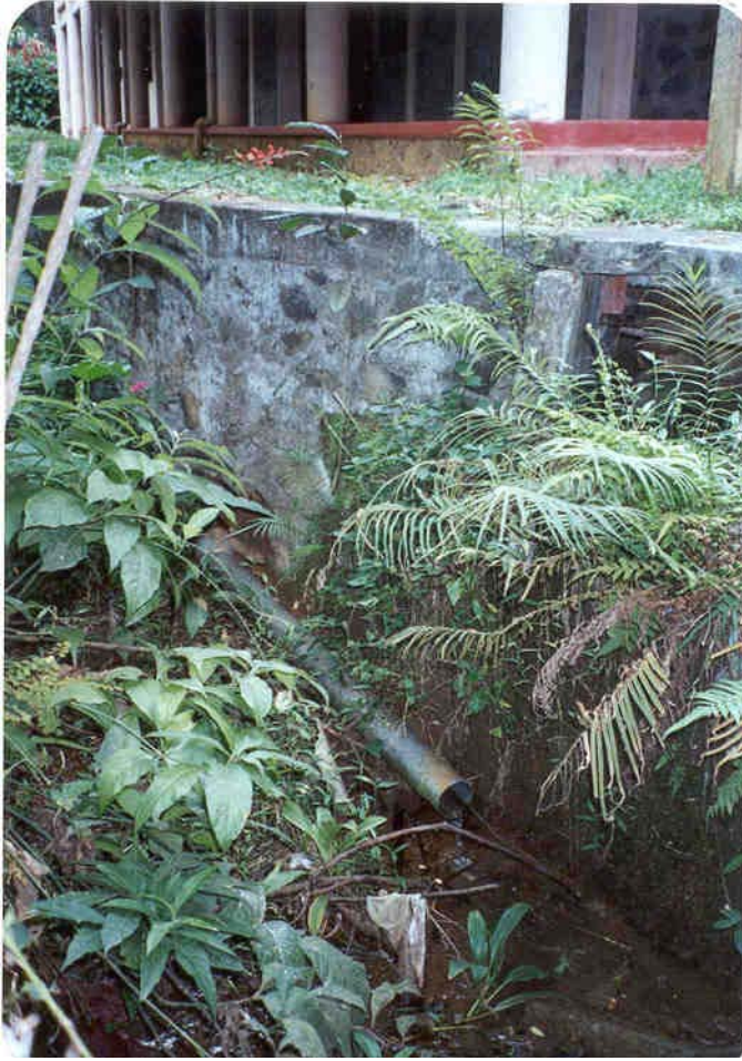
Plate 3-57. The discharge point of the PGIA anaerobic filter
