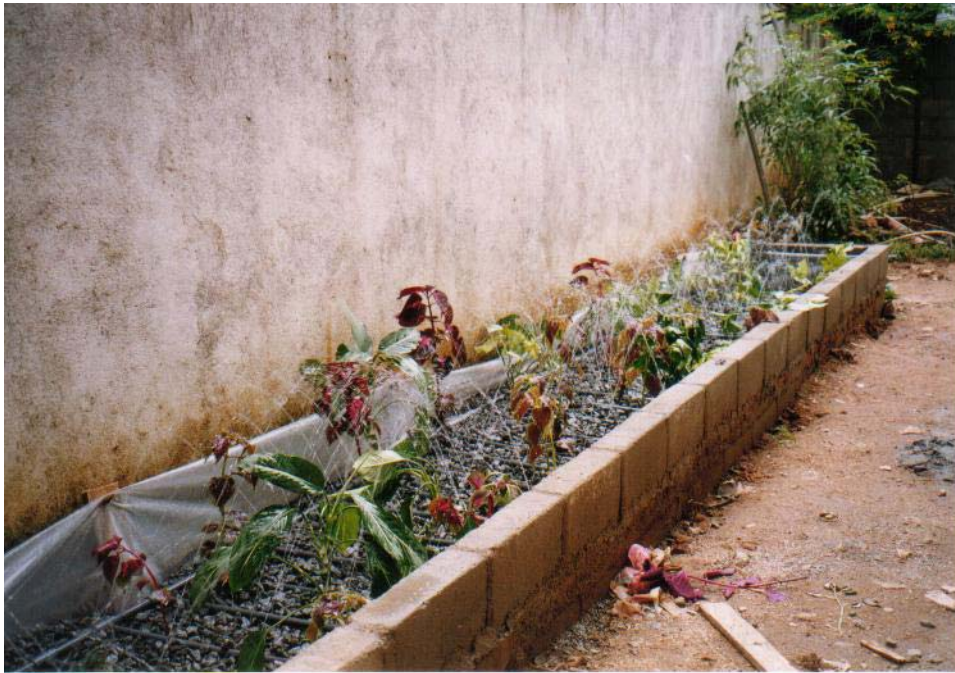
Plate 3-28. The VFPGF unit immediately after commissioning.
