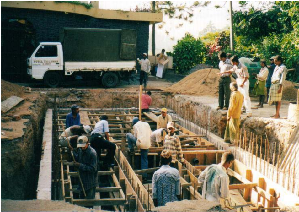
Plate 3-16. The combined septic tank – anaerobic filter unit during construction under a parking area.
