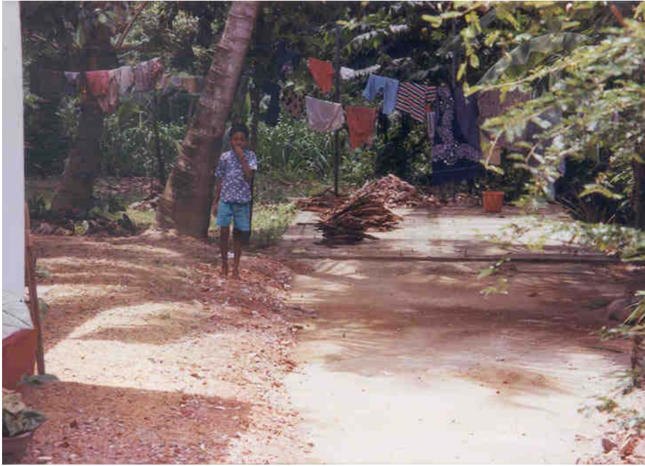
Plate 3-40. The anaerobic filter unit at Ranpokunugama after commissioning
