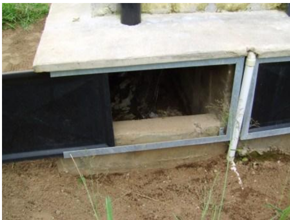
Figure 5. Close-up of one of the vaults with its sliding door partially open. The urine-diversion pipe is clearly visible on the right.
