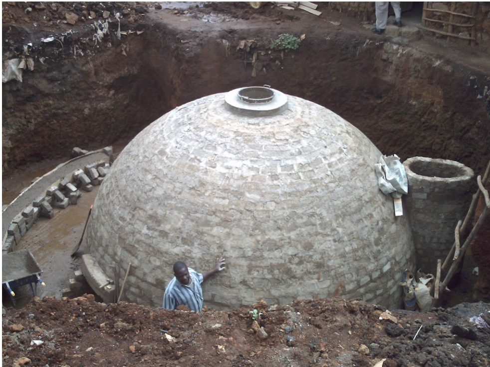
Figure 2. Anaerobic digester which receives all the wastewater from the sanitation block. The biogas generated in the digester is used for cooking.
