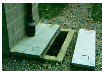
Figure 2. An alternating twin-pit VIP latrine. Each of the two pits has its own 100-mm diameter vent pipe with a fly screen at its top. The external pit cover slabs are only weakly mortared so they can be easily removed when the pit is to be emptied:
