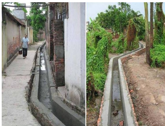
Low-cost combined drainage at Lai Xá, Vietnam
