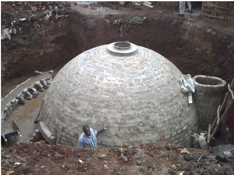
Figure 2. Anaerobic digester which receives all the wastewater from the sanitation block. The biogas generated in the digester is used for cooking.
