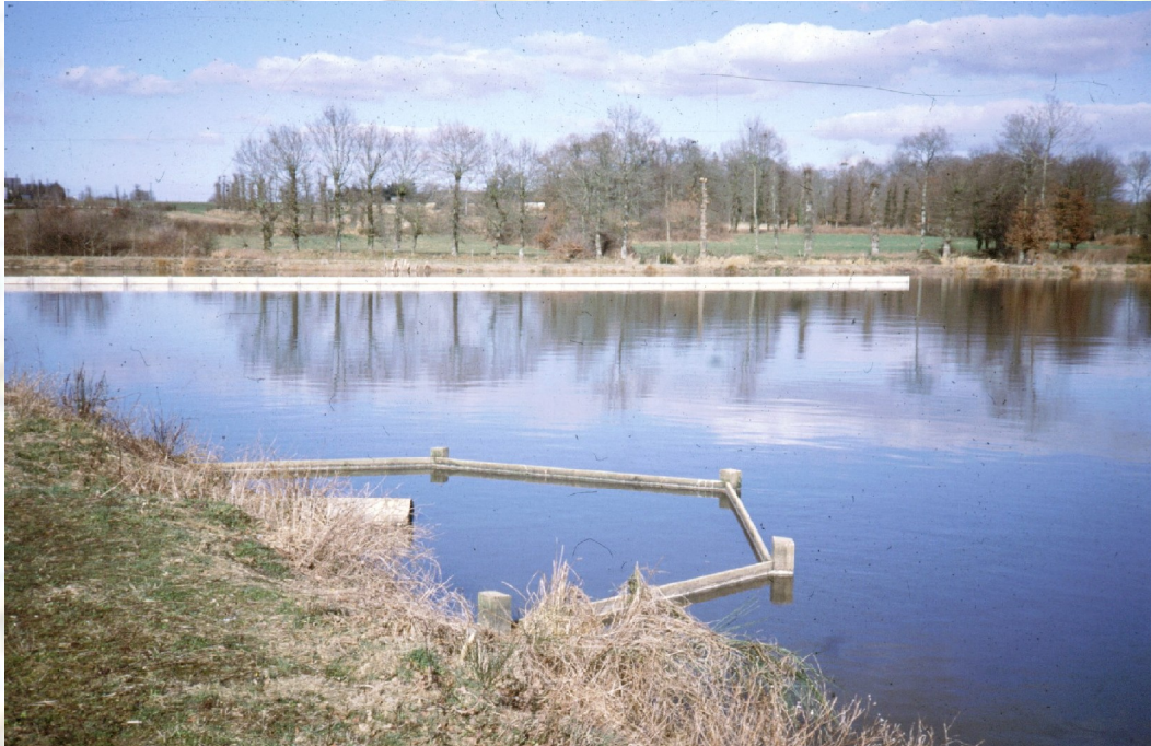
Figure 4.11. Scum baffle at the inlet of a primary facultative pond in France
