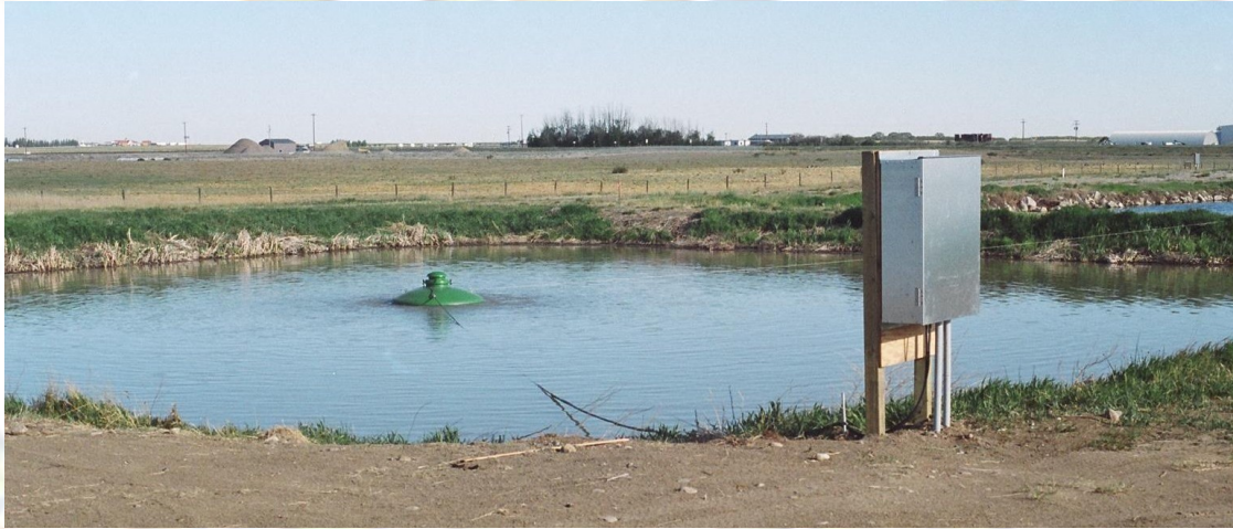
Figure 4.6. Floating electric mixer/circulator pump on a facultative pond in Canada Photograph courtesy of Solar Sunset Systems Ltd
