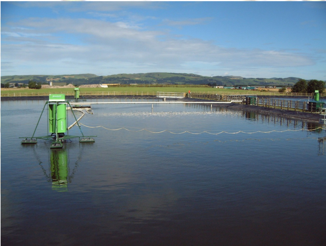
Figure 4.7. The primary Aero-fac® lagoon at Errol, by Dundee, showing the wind-powered aerators Photograph courtesy of Ms Michelle Johnson, School of Civil Engineering, University of Leeds
