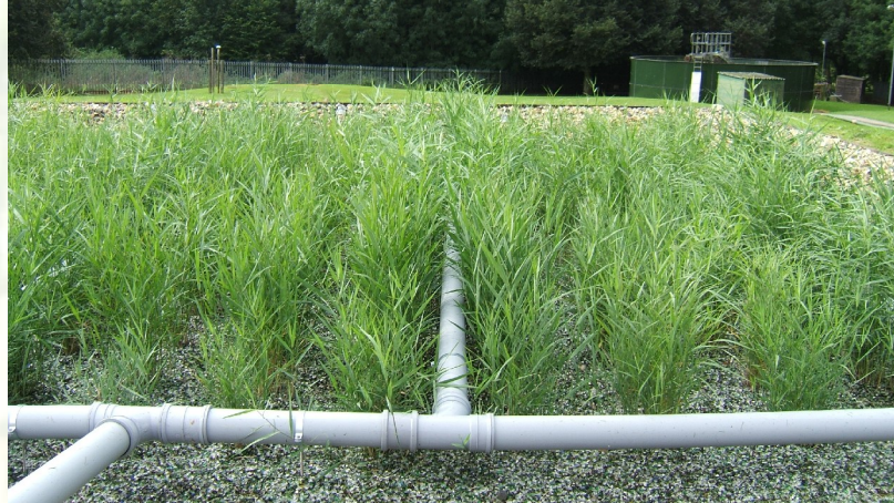
Figure 3.7. Bed medium of recycled glass in the VF-CW at Bernard Matthew Ltd, Great Witchingham, Norfolk Photograph courtesy of Dr Nigel Horan, School of Civil Engineering, University of Leeds
