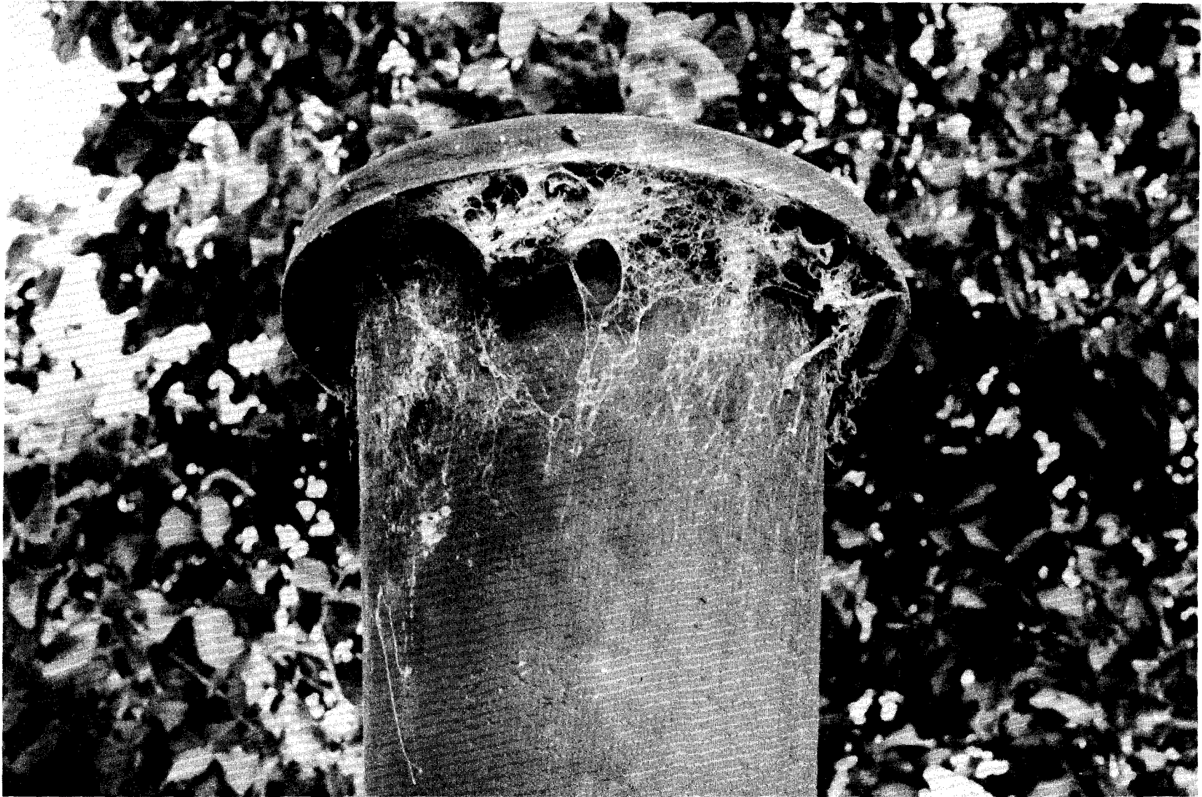
Figure 6: Cobwebs at the top of a vent pipe.
