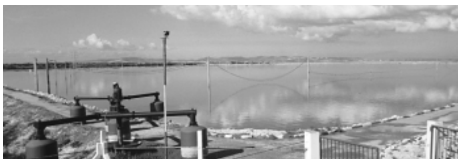
Figure 5.3 Primary facultative pond at Cotière Nord (one of the standby aerators, left, has been removed for repair)
