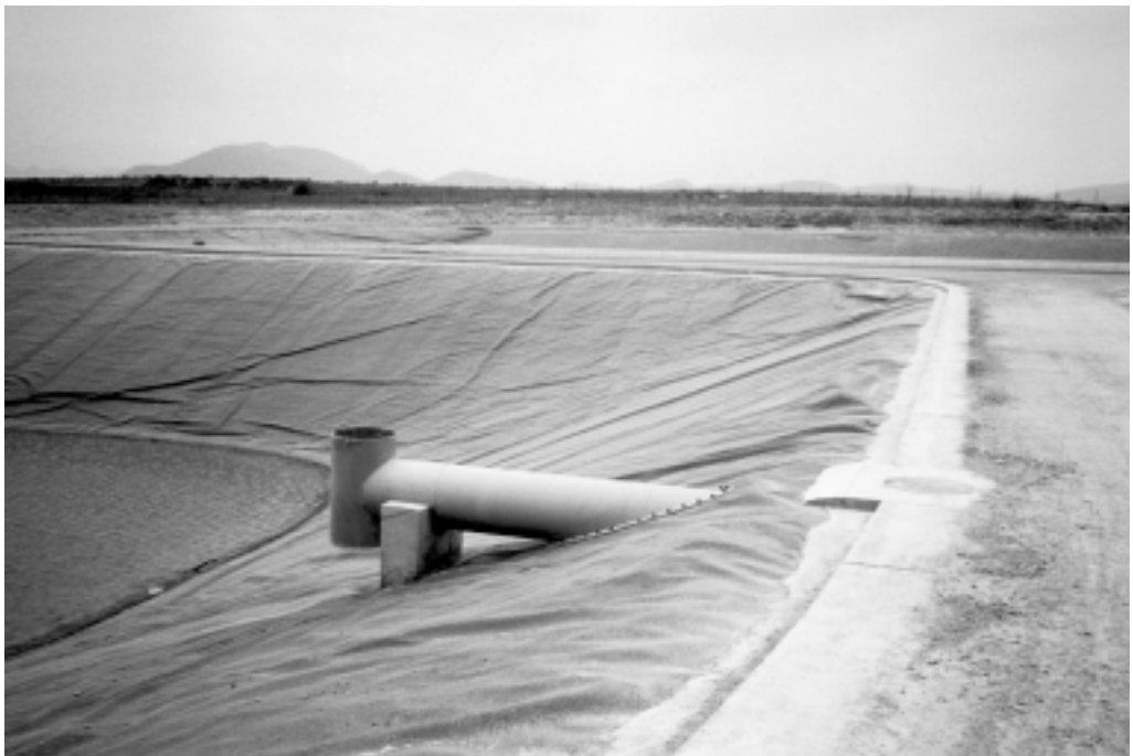
Figure 5.3 Anaerobic pond lined with an impermeable plastic membrane.
