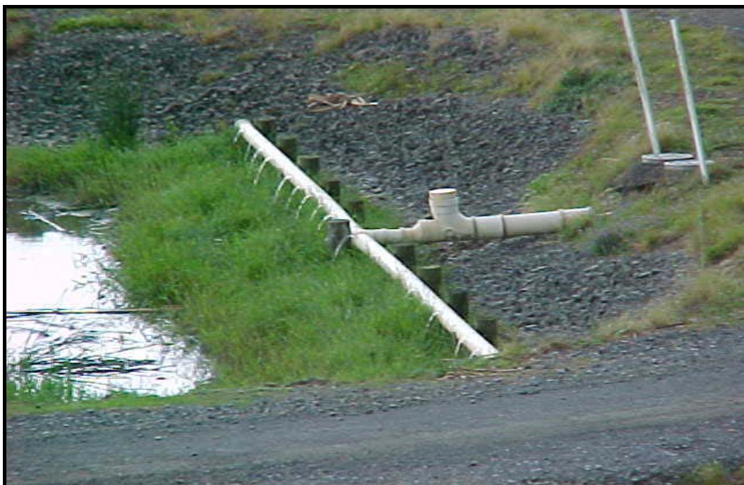
Figure 4-7 An inlet manifold used on a surface flow wetland system
