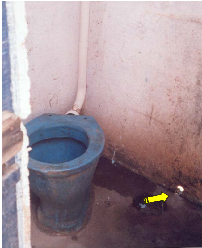
Plate 5.1. – Opening to allow sullage to drain from the units
