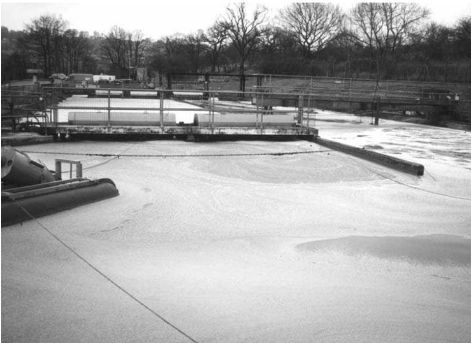
Fig. 32.6 Foam can be managed to an acceptable level and retained on the surface of the aeration tank.
